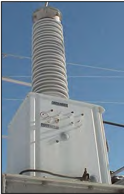
Potential Transformer in switchyard.
