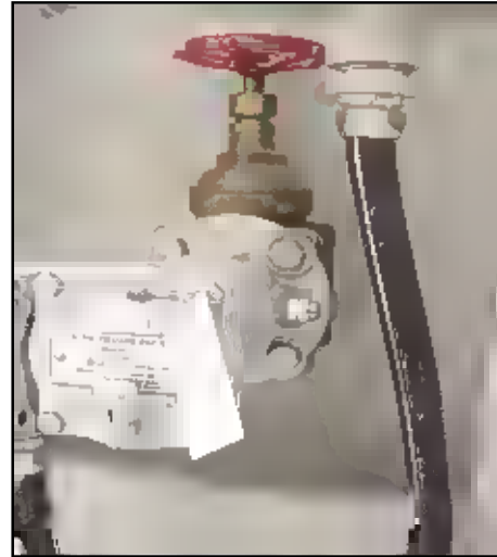
Figure 32 – Photograph of a Sudden Pressure Relay.
