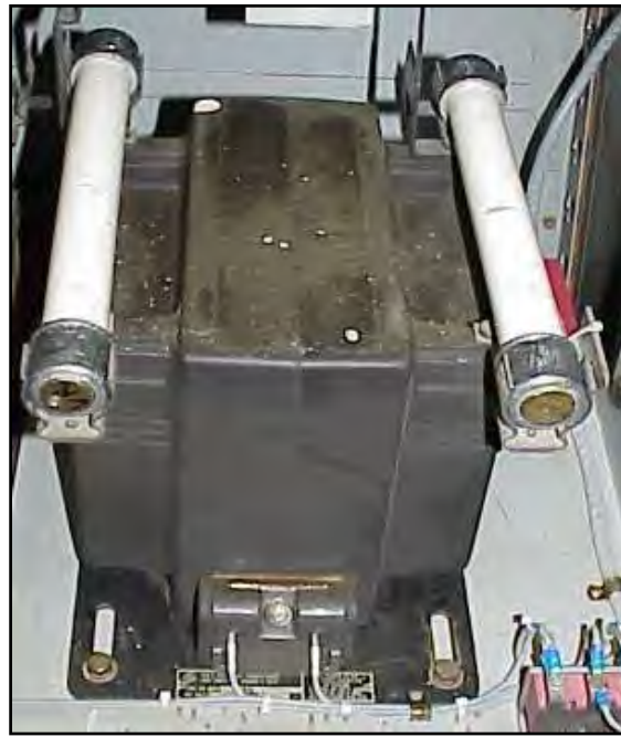
Inside Potential Transformer with Fuses.
